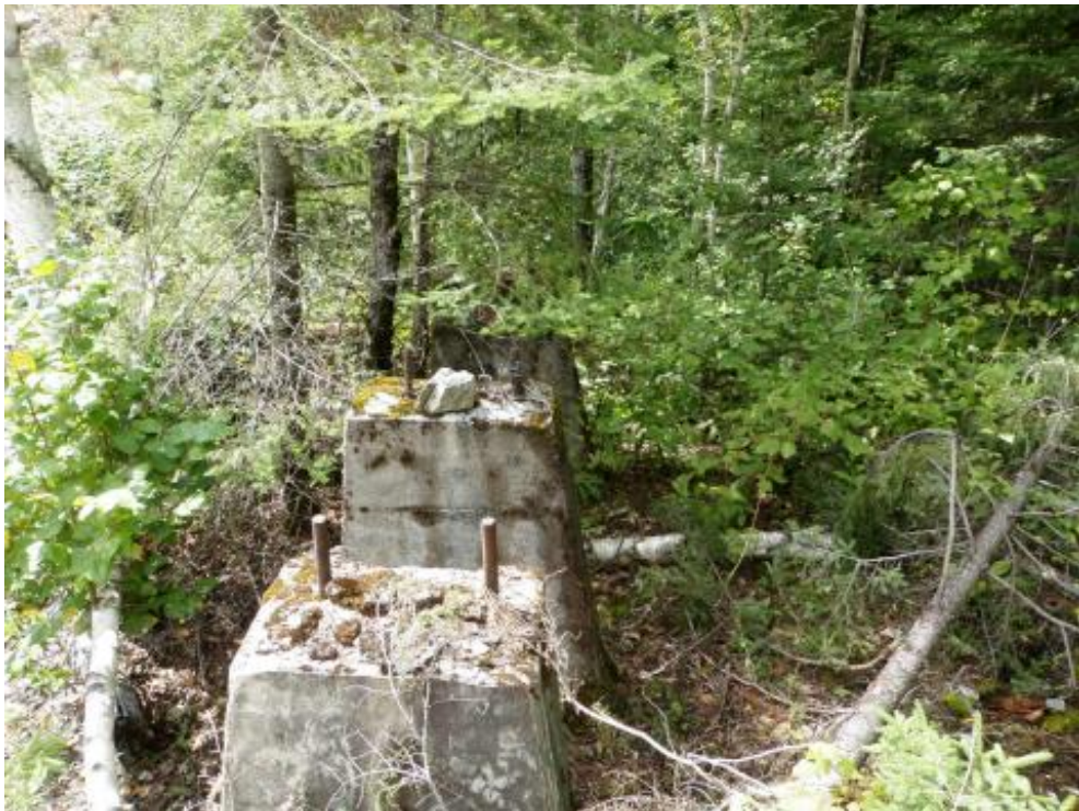
Figure 17: View of Concrete Pedestals in the Central Area of the Stamp Mill (View West)
