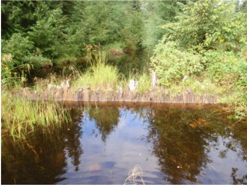
Figure 31: Timber Crib Dam Structure along Secondary Channel in Stream Valley (View West)
